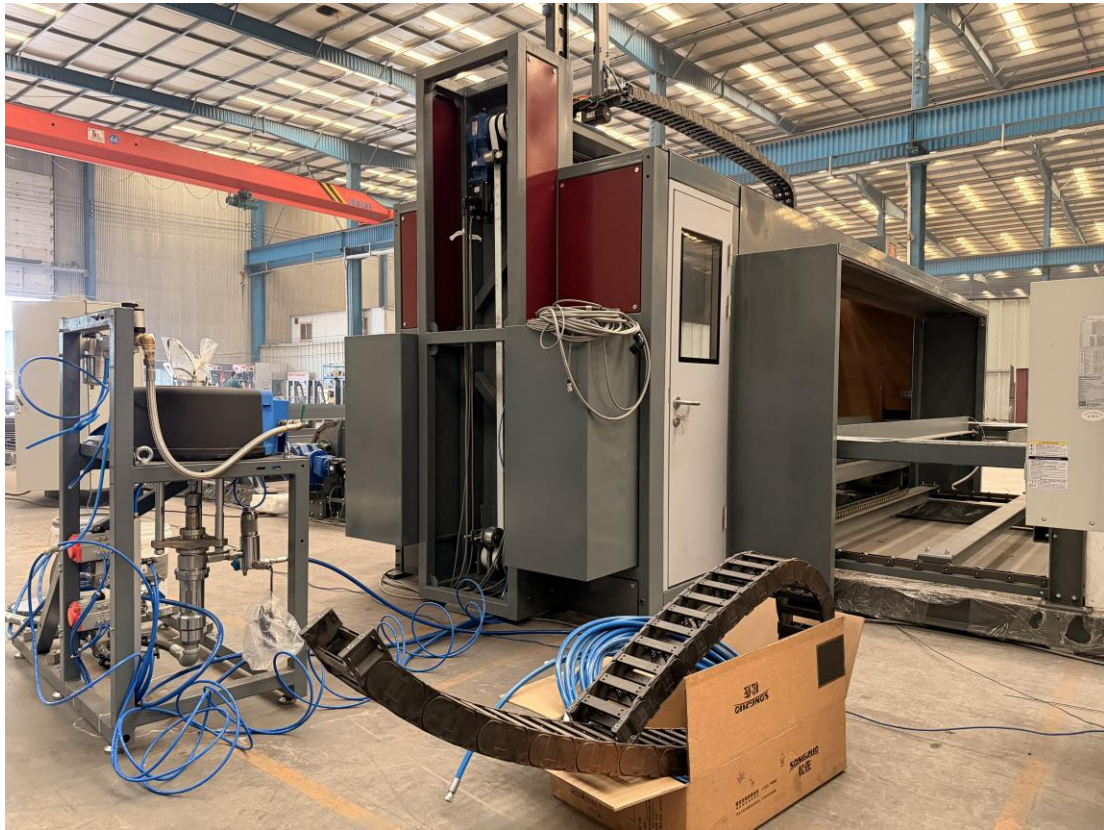
Spray booth and spray pump
