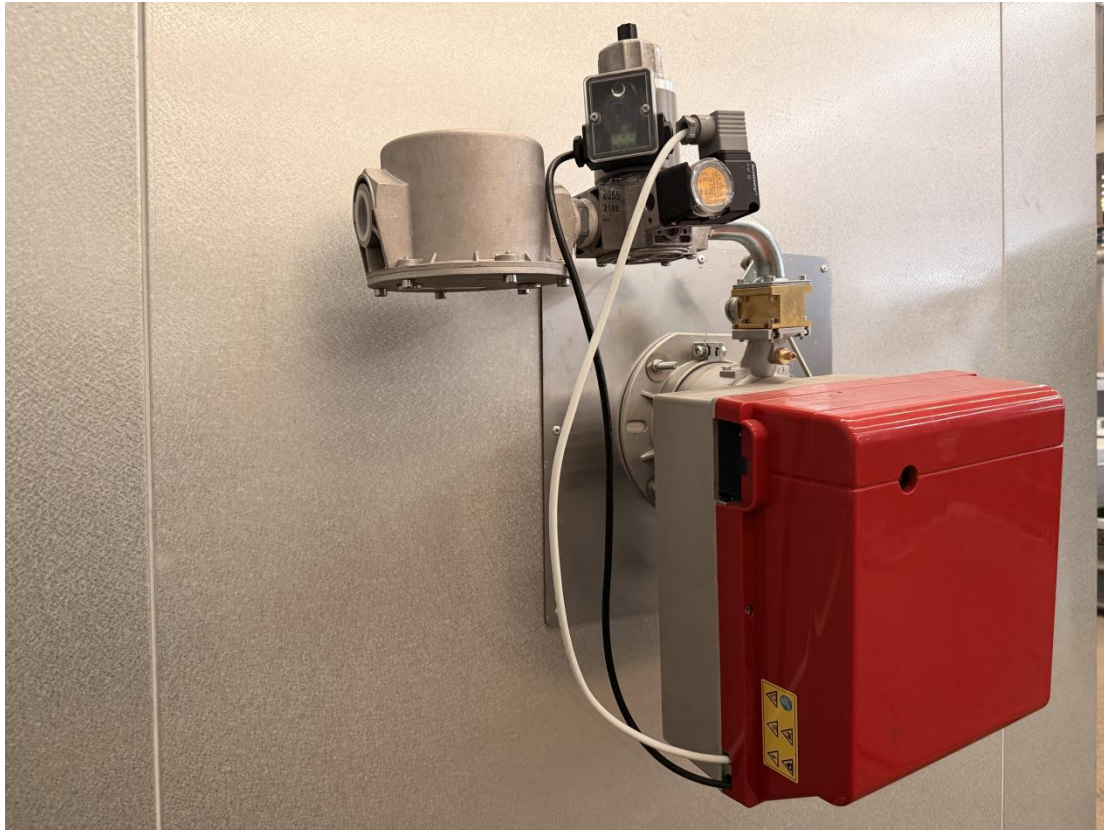
Hot air furnace
